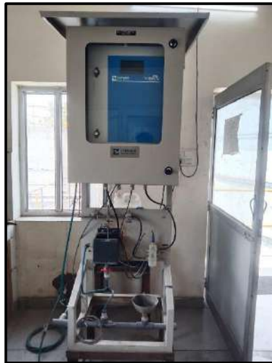
Online Continuous Monitoring System
